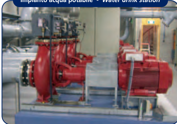
Impianto acqua potabile - Water drink station
